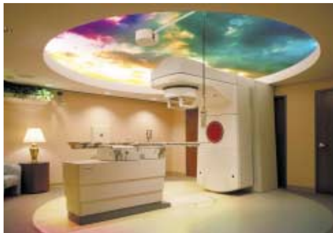
Design of the linear accelerator room at Baylor Healthcare System in Irving, Tex., provides a soothing and beautiful surrounding for patients undergoing radiation therapy.
