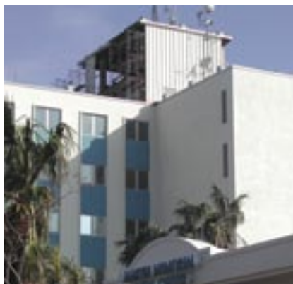
The north elevator tower of Martin Memorial Medical Center was damaged during Hurricane Frances in Sept. 2004, limiting access to floors two through six.
